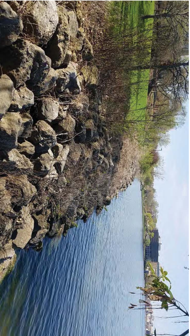
The northeastern half of the shoreline is lined with large boulders on a steep slope.
