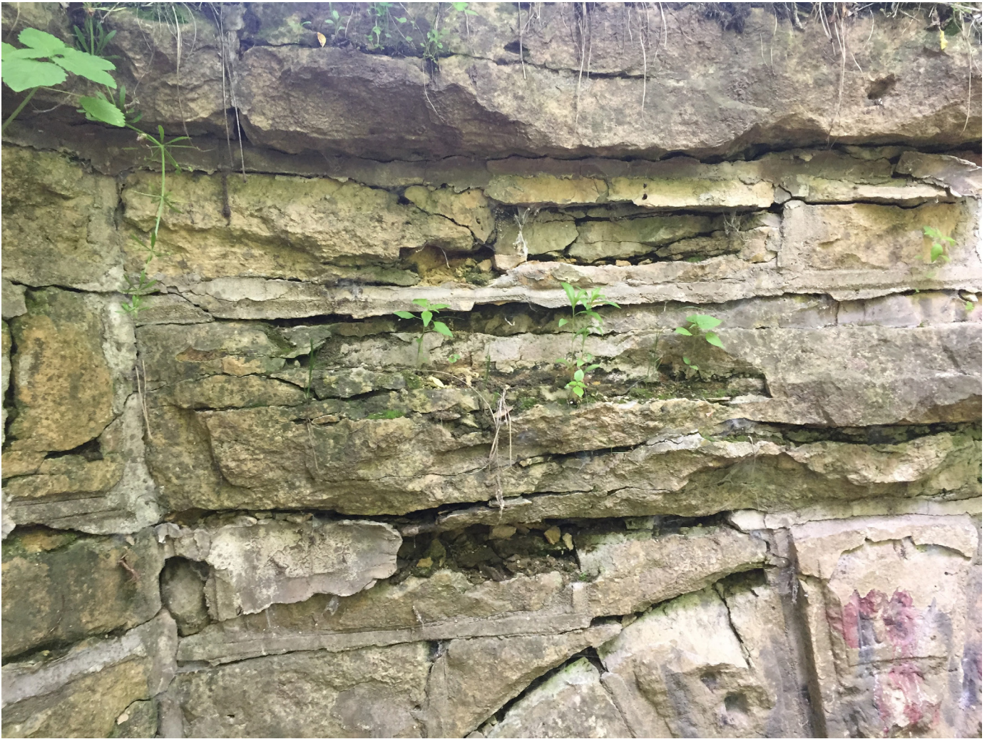
Figure 4: General disintegration of stone above the arch.
