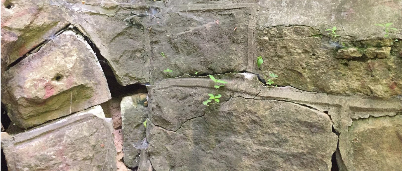
Figure 5: Right side of arch deflection and beginning of collapse.
