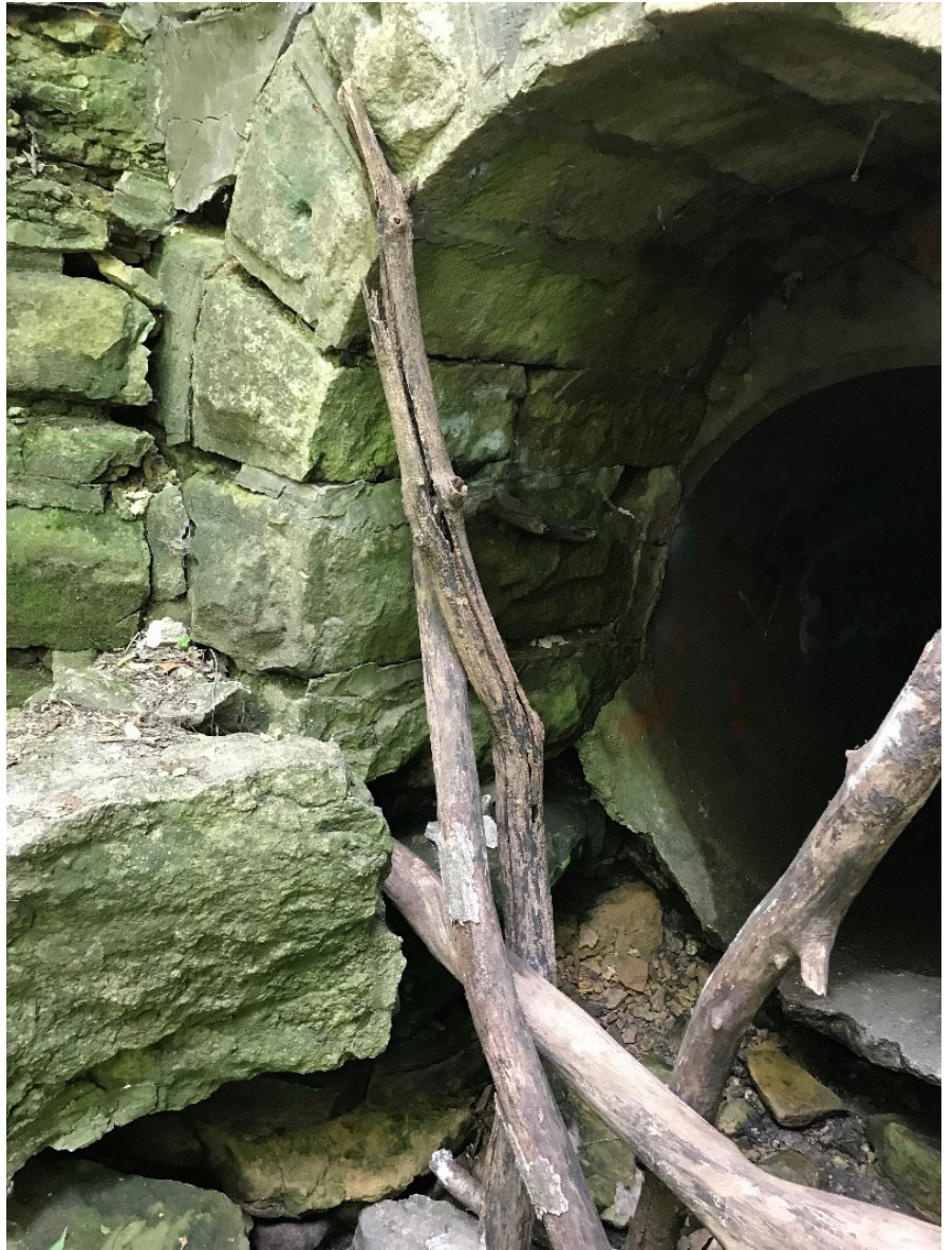
Figure 8: Undercutting of the arch at left and 2-3' stone construction depth to the intact concrete culvert that conveys stormwater under the bike path.
