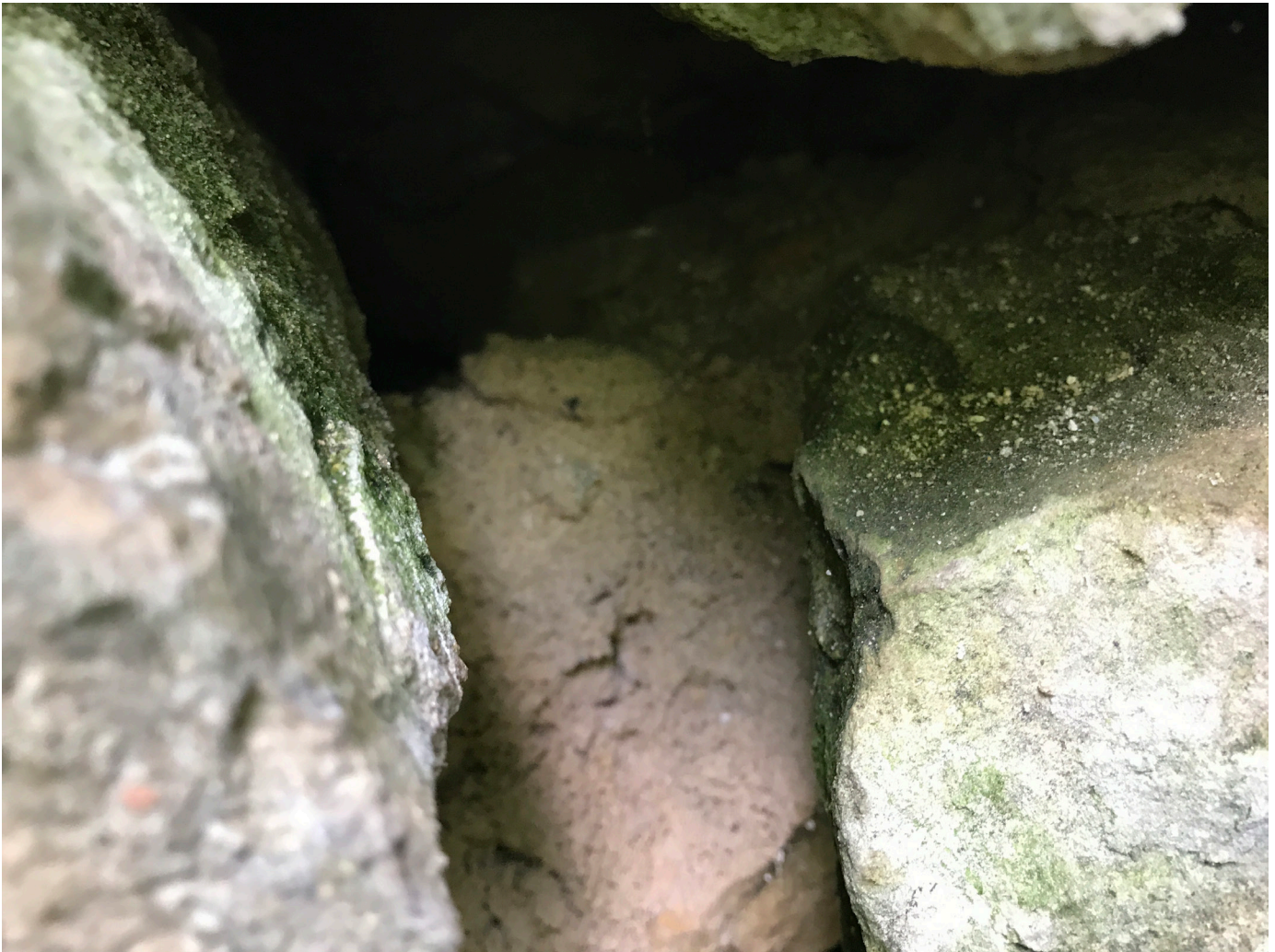
Figure 12: Degradation of the arch stones deeper in the wall is visible from the open joints where the arch has come out of alignment due to settling at the base at the right.
