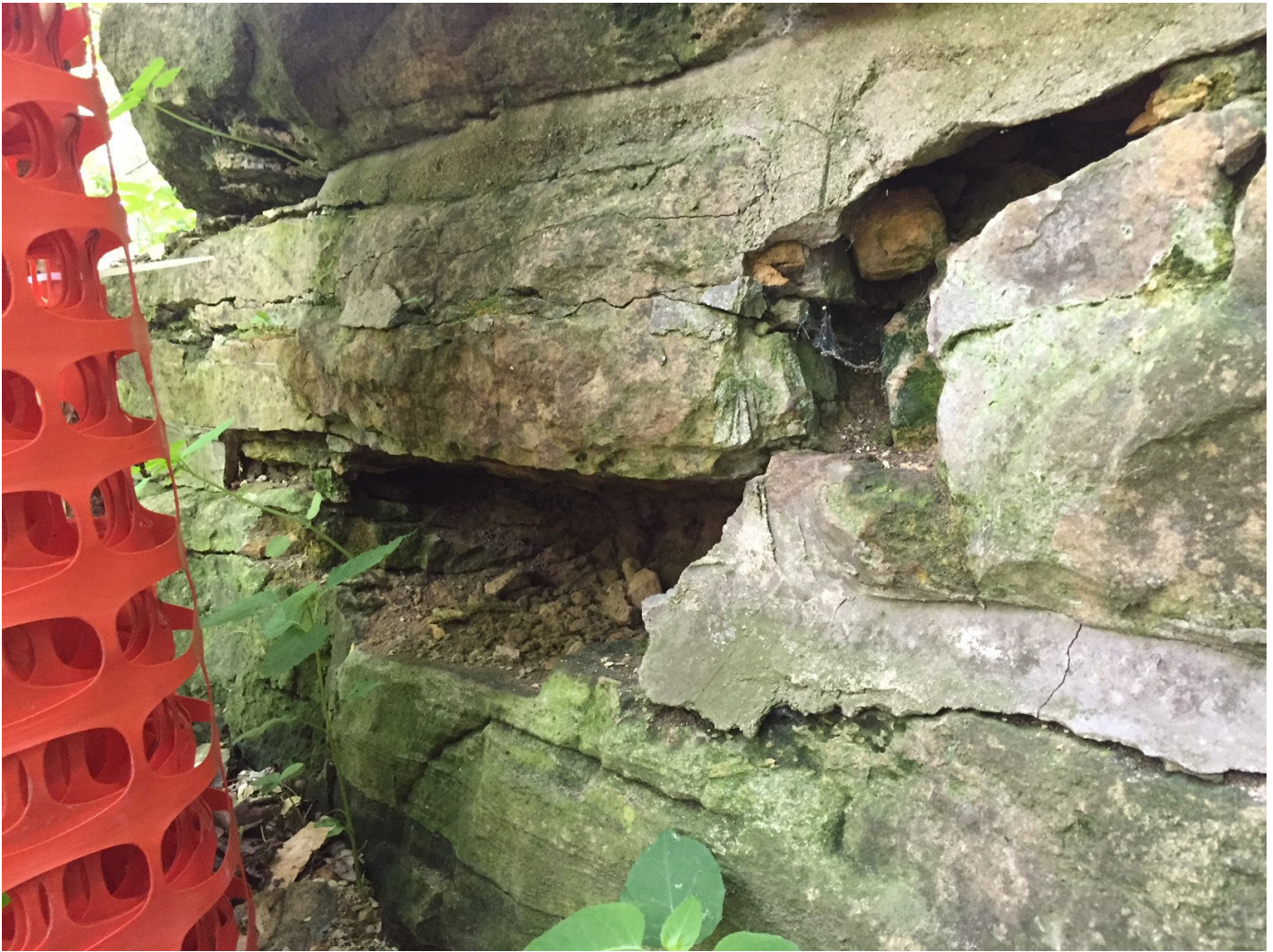
Figure 11: Degradation of the sandstone at the wing walls is most advanced at the face.
