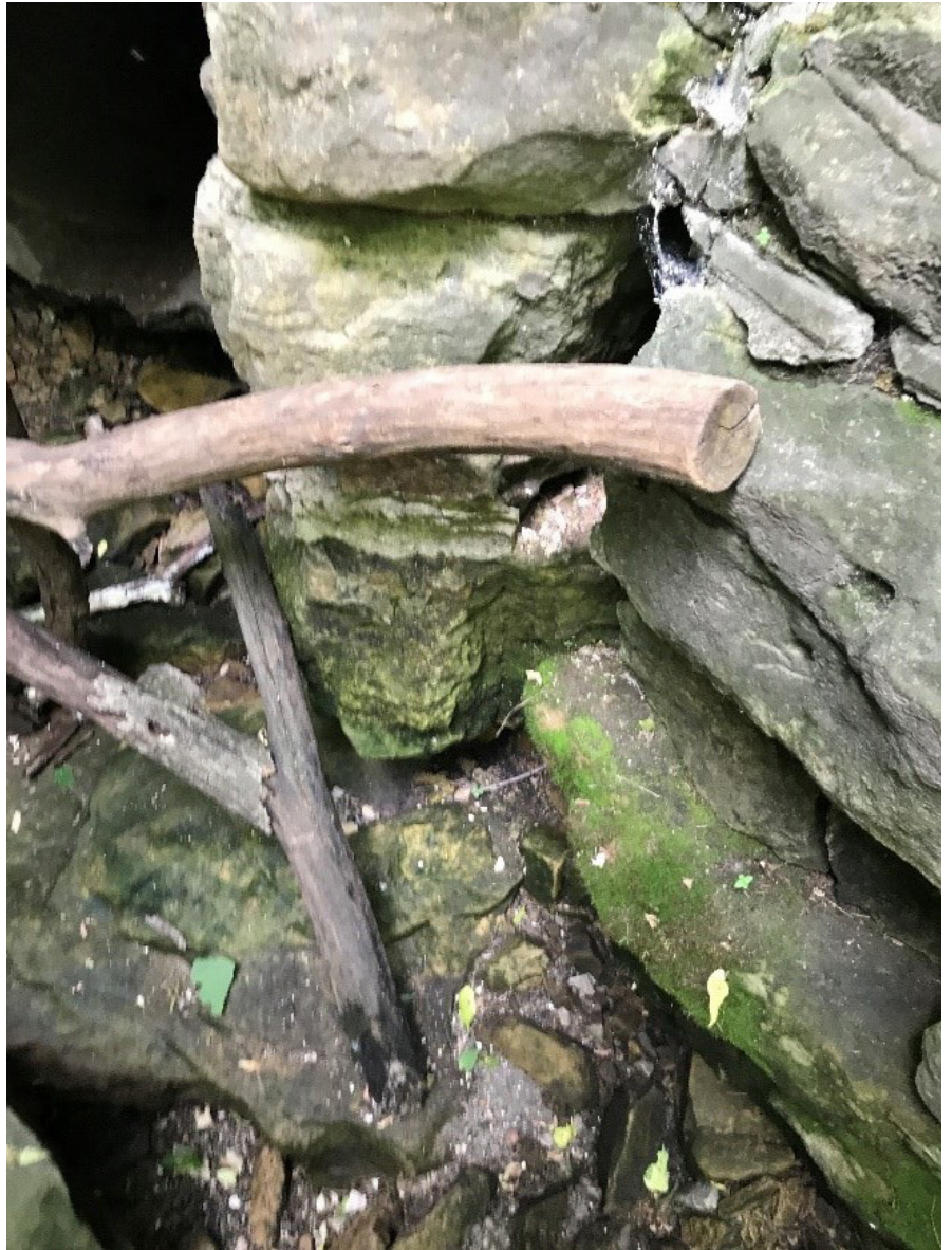
Figure 6: Arch bearing condition at right.
