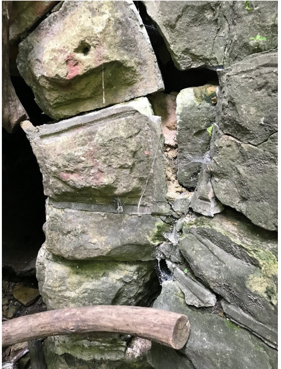
Figure 10: Degradation of the sandstone at the wing walls is most advanced at the face.
