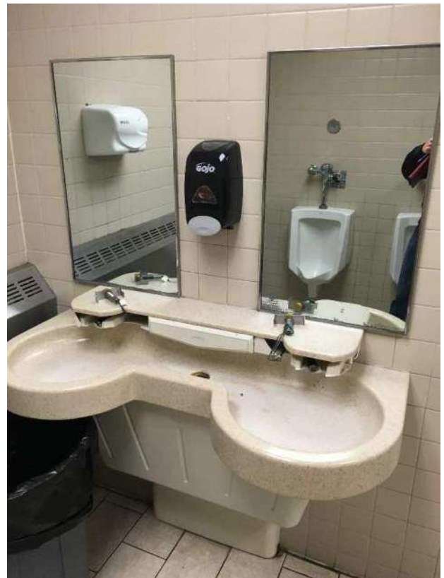
Sinks in main restroom area
