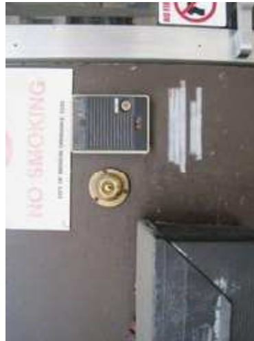
Figure 293 Intercom Device- Exterior
