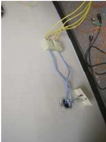
Figure 288 IT Cabling – Voice/Data
