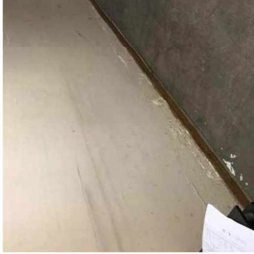
Figure 54 – Plaster over cmu wall damage
