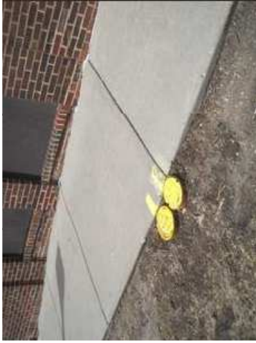
Figure 466 - Gas Service - Exterior
