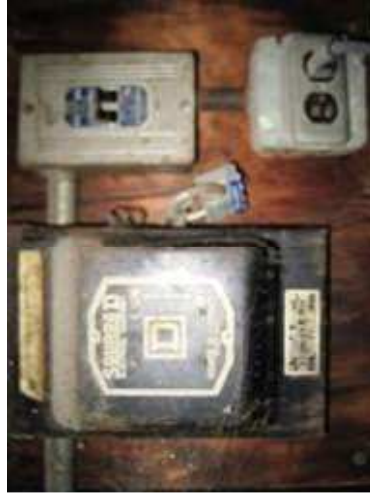
Figure 206 Main Electrical Disconnects – Main Level
