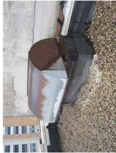
Figure 181 - Parking Garage Vent Discharge
