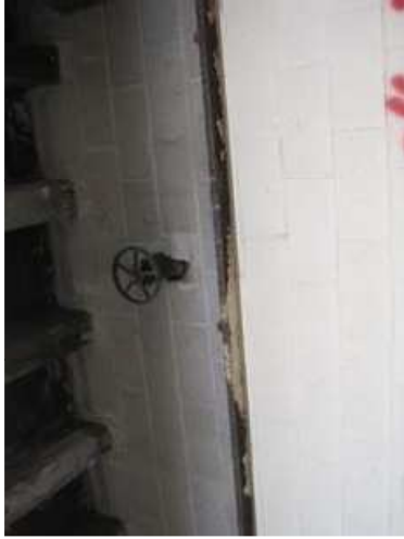
Figure 176 - Steam Valve Boiler Isolation
