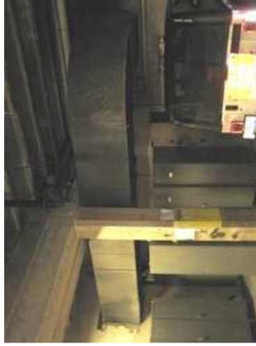
Figure 180 - Combustion Air Duct
