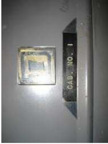
Figure 210 Electrical Panel No. 1 - Maintenance Area
