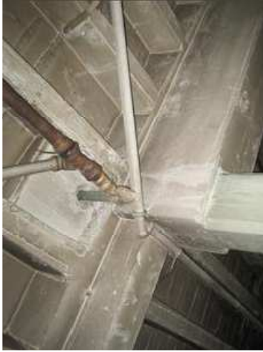
Figure 447 - Sanitary to Floor Drains Above
