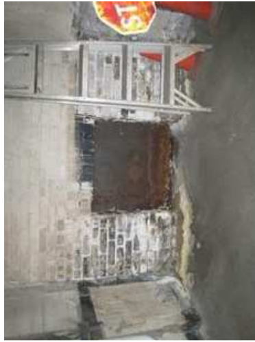
Figure 172 – Lower Level Exhaust
