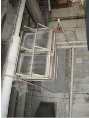
Figure 168 – Combustion Air Duct
