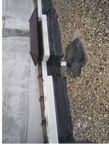
Figure 184 – Parking Garage Vent Discharge
