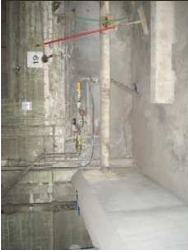
Figure 402-Water Service Meter – Inside
