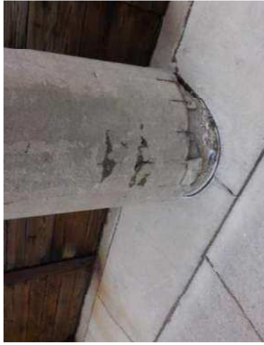
Column base deterioration
