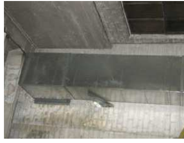
Figure 173 – Lower Level Exhaust
