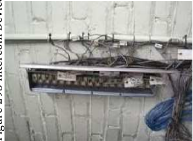
Figure 296 Abandon Telephone Wiring
