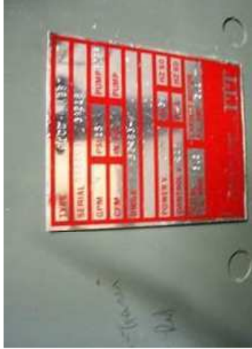
Figure 112 – Condensate Tank Nameplate
