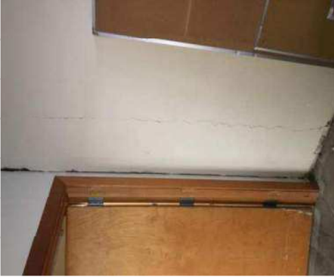
Figure 59 - Interior wood door & Gypsum
