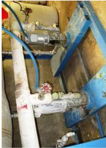
Figure 107 – Boiler Feedtank Pumps
