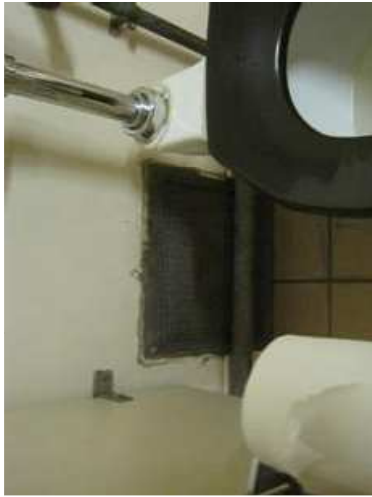
Figure 139 – Restroom Exhaust Grille
