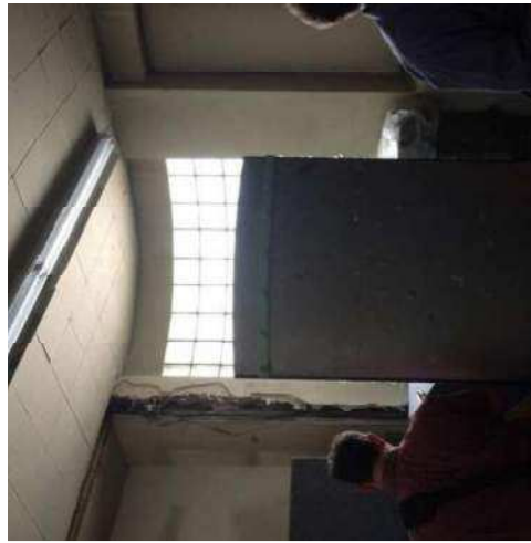
Figure 55 – Plaster damage @ glass block
