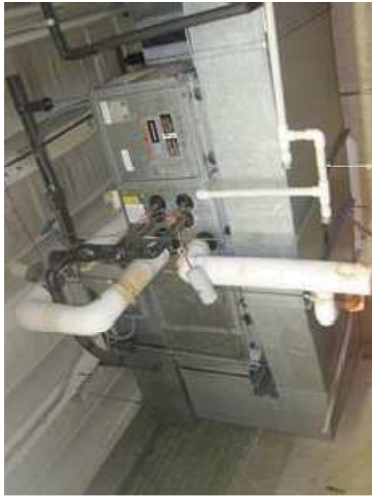
Figure 128 -- AHU Soften Water Tank
