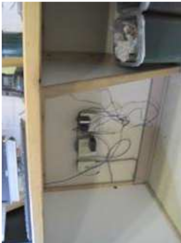
Figure 299 Office Data Cabling
