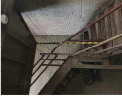
Figure 24 – NE Stair Headroom issue
