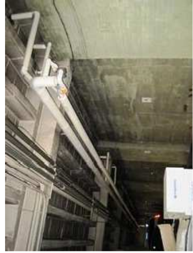
Figure 147 – Steam and Condensate Piping
