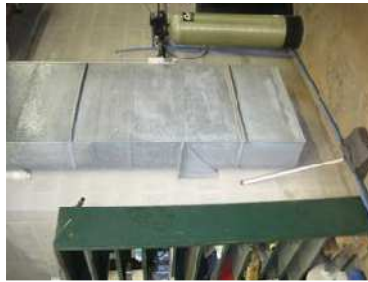
Figure 178 - Boiler Combustion Air Duct
