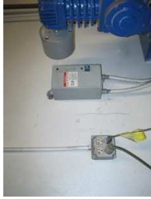
Figure 434 - Power to Compressor
