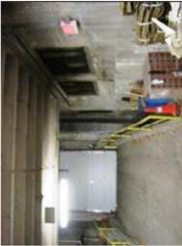
Figure 273 – Lighting in Parking Garage Areas
