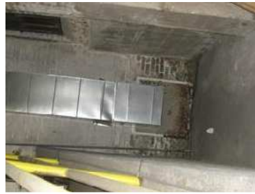
Figure 174 – Lower Level Exhaust
