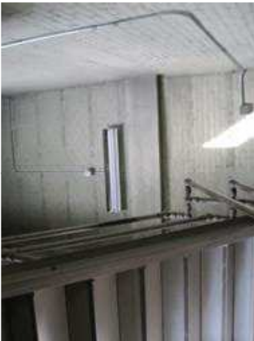
Figure 272 – Stairwell Lighting with Occupancy Sensor
