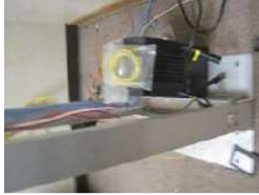
Figure 285 UPS IT Rack
