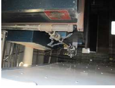
Figure 158 – Makeup Air Unit
