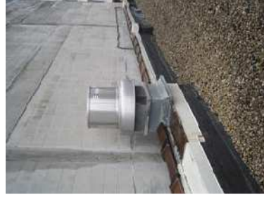
Figure 187 – Roof Exhaust Fan
