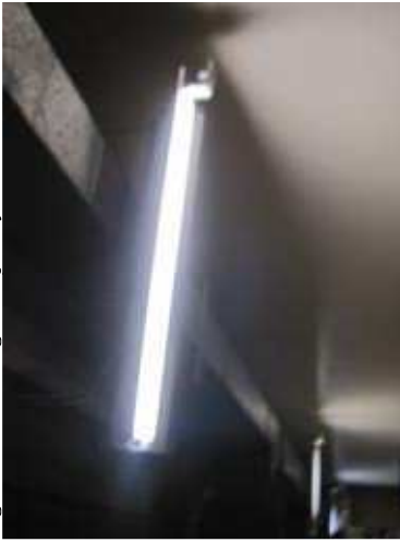
Figure 258 Lighting with Occupancy Sensor
