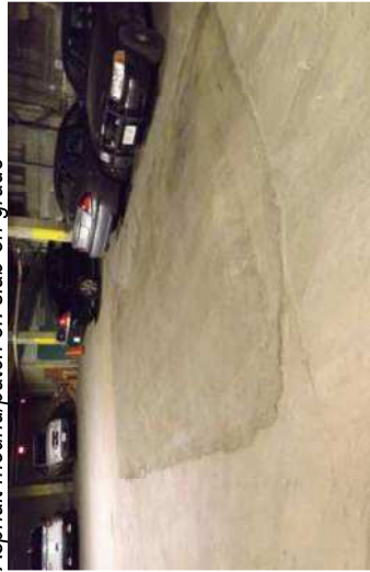
Asphalt mound/patch on slab-on-grade
