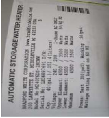
Figure 411 - Water Heater – Nameplate
