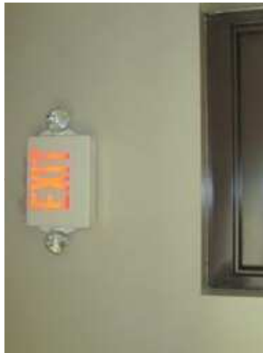
Figure 304 Exit Sign/Emergency Lighting (Battery)
