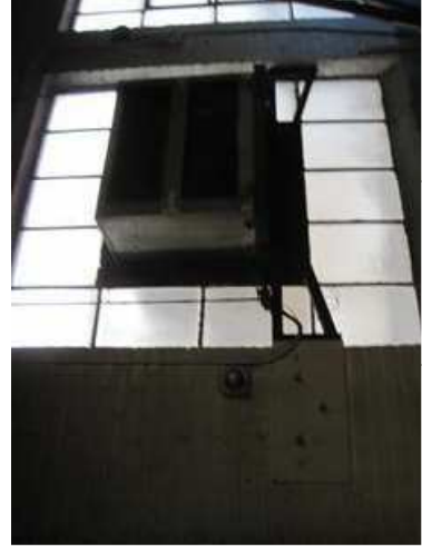
Figure 138 -- Room AC Unit
