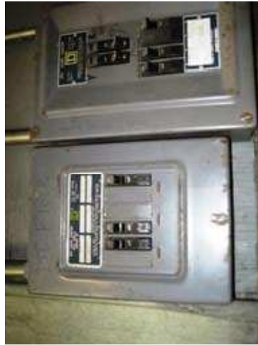
Figure 205 Electrical Sub Panels
