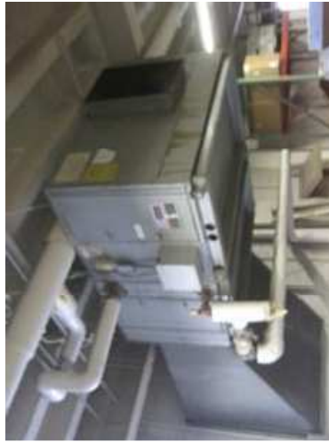
Figure 142 – Make-up Air Unit
