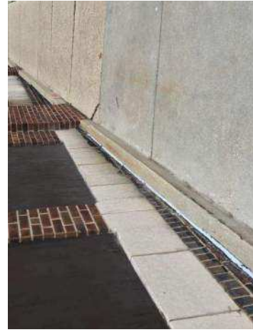
Caulk joint failing at brick and sidewalk
