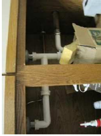
Figure 407 - Kitchette Sink Area
