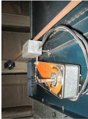
Figure 161 – Electric Actuation on Unit
