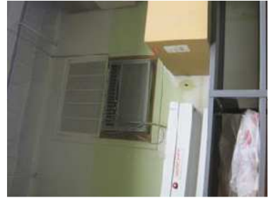
Figure 135 -- Room AC Unit
