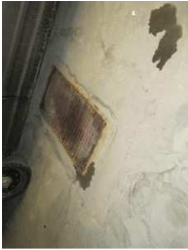
Figure 457 - Trench Drains - Wash Area
