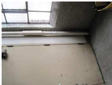
Figure 439 - Piping at Exterior
