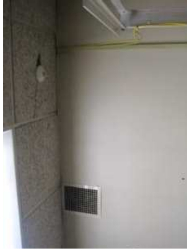
Figure 134 -- Room Return Grille
