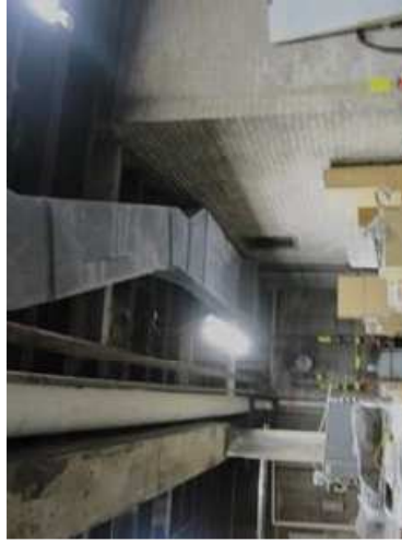
Figure 179 - Combustion Air Duct
