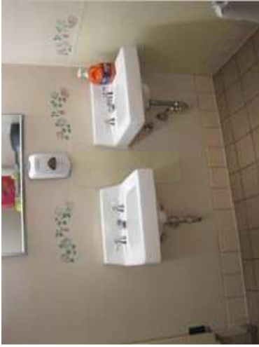
Figure 420 - Women's Wash Sinks
