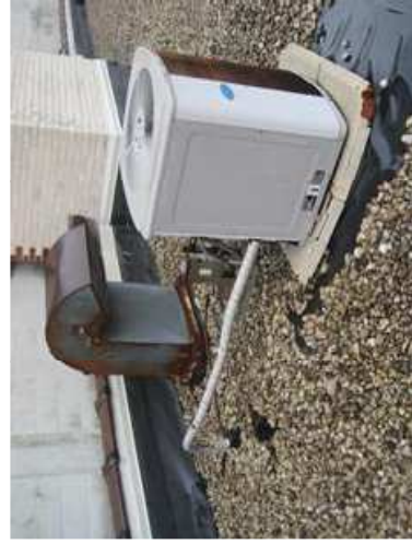
Figure 183 - AHU-1 Air-Cooled Condensing Unit
