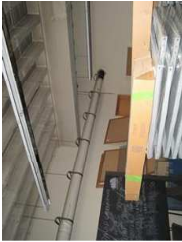
Figure 438 - Sanitary Piping through Storage Area
