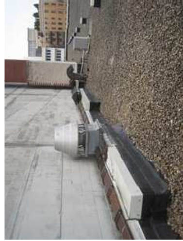
Figure 182 - Exhaust Fan Parking Garage
