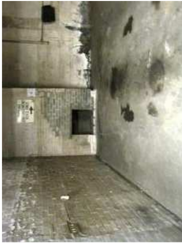
Figure 167 – Lower Level Exhaust
