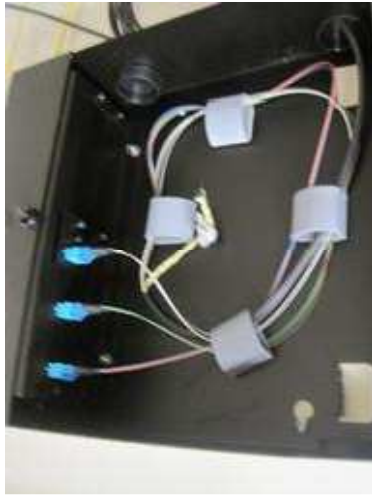
Figure 289 Patch Panel – Phones
