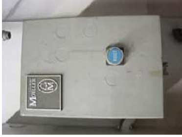
Figure 250 Exhaust Fan Starter
