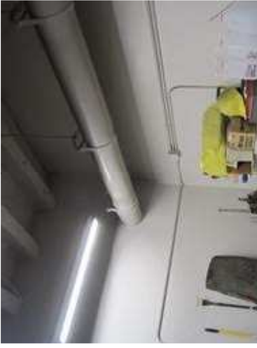
Figure 268 Lighting with Local Switch
