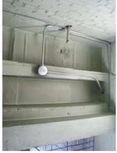
Figure 271 - Occupancy Sensor - Storage Area
