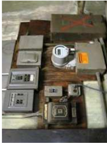
Figure 202 Main Electrical Meter – Main Level
