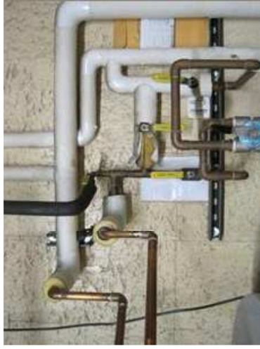
Figure 414 - Plumbing Mixing Valve
