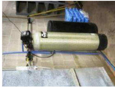
Figure 467 - Softener to Boiler
