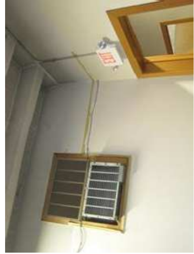
Figure 136 -- Room AC Unit
