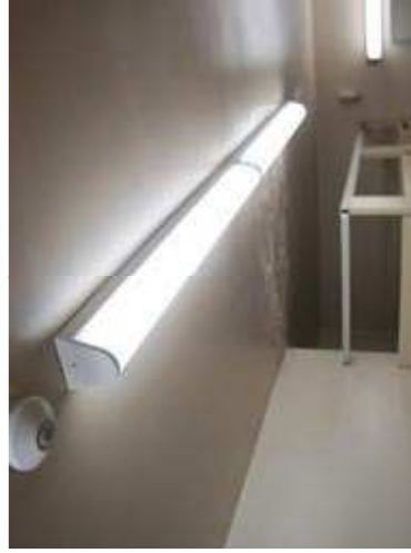
Figure 263 Lighting – Women's Restroom
