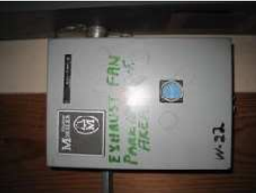
Figure 227 Exhaust Fan - Starter
