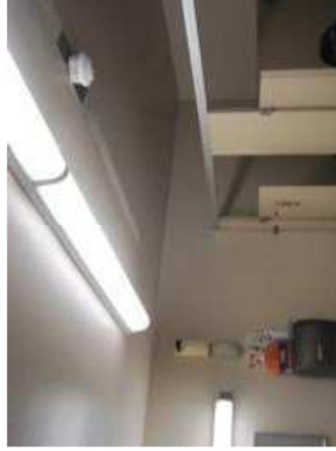
Figure 262 Lighting – Men's Restroom
