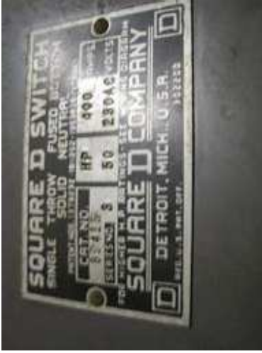
Figure 207 Main Distribution Switch Identification
