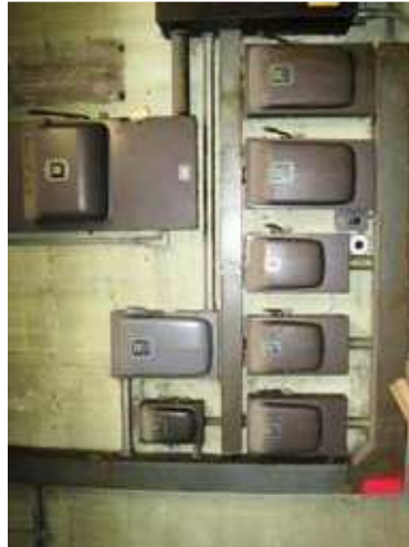
Figure 204 Main Electrical Disconnects – Main Level
