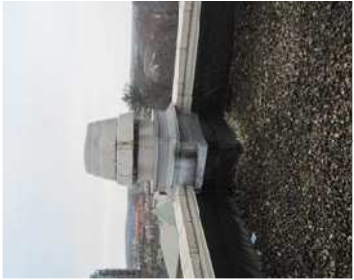
Figure 191 – Roof Exhaust Fan
