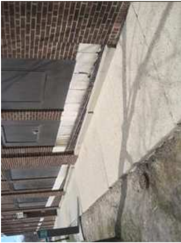
Figure 401 - Water Service Entrance – Outside
