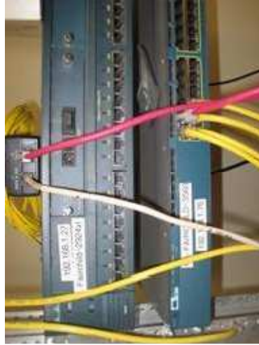
Figure 287 IT Server - Patch Cords
