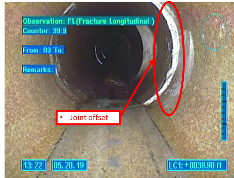
Sanitary sewer main south of Brody.
