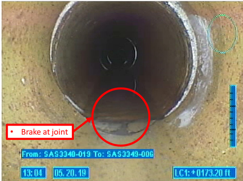
Sanitary sewer main south of Brody.
