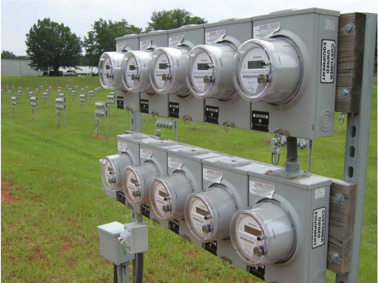
Figure 9-2 Typical rack of ten meters shown in the western part of the Itron meter farm.
