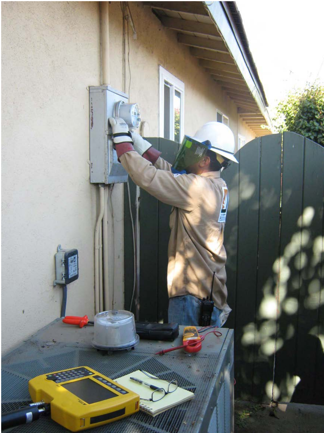
Figure 9-13 SCE meter technician replacing existing Smart Meter with specially programmed meter for residential measurements.
