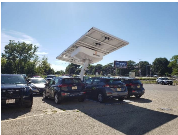
EVs charging at a solar-powered charger.
